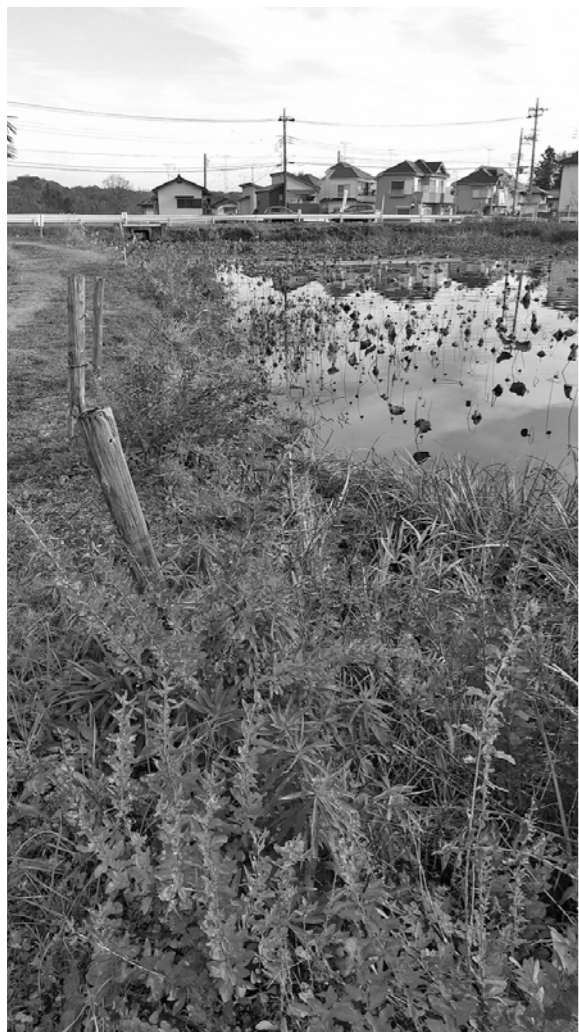
浸食、崩落が進む天沼 = R3.12.12
